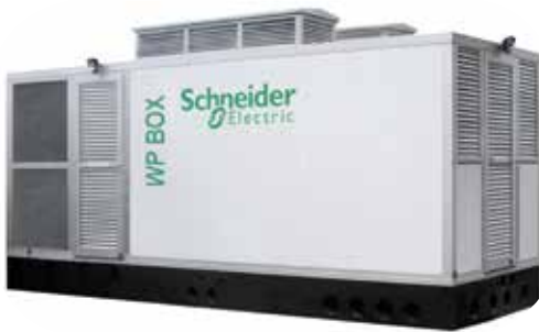
Wind Power Box - Transformer Substation
