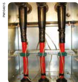
Connectors.MV Cable compartment
