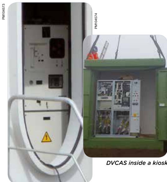
DVCAS inside the wind turbine
